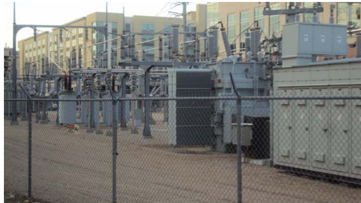
Grove Street Substation.
