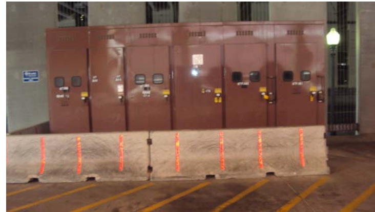
Switch station located in the St. Luke's Boise parking garage.
