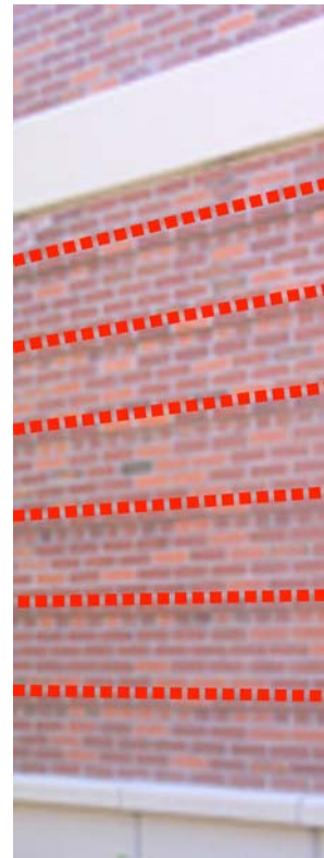
Recessed brick creates interest at exterior walls at the St. Luke's Boise facility.
