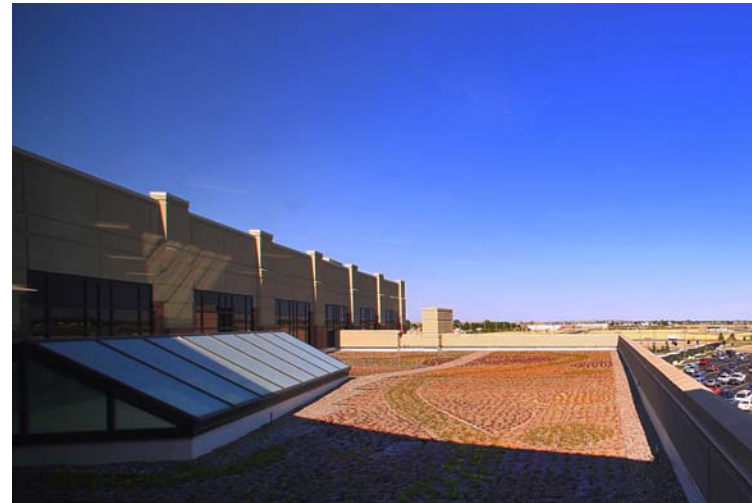
Vegetated roof helps to reduce runoff and heat island effects at St. Luke's Magic Valley.
