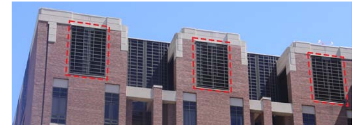
Mechanical grilles are used and arranged in the same fashion as glazing to break up and divide exterior walls.
